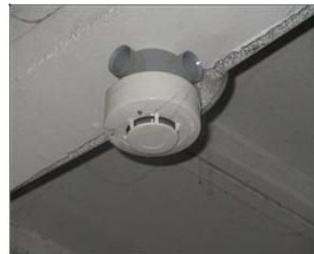
Photo of fire safety equipment Smoke detector.JPG
