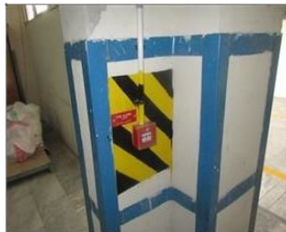
Photo of fire safety equipment Fire alarm.JPG
