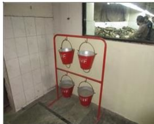
Photo of fire safety equipment Fire buckets.JPG
